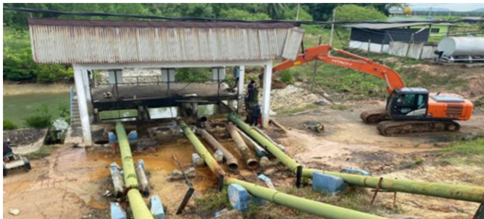
Seawater Intake system
